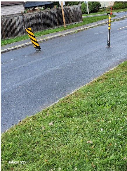
Although only recently installed, the traffic pylons are already showing signs of wear.
